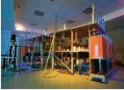
Lightning current generator
